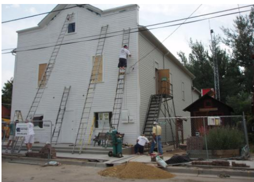
Our museum remains behind a chain link fence as workers complete their renovation of Left Hand Grange last summer.
